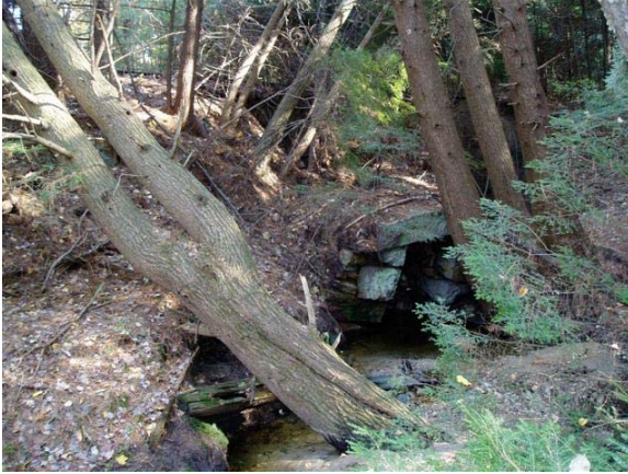
Figure 44: Culvert No. 42.37 Collapsed Culvert
