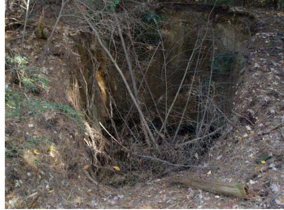
Figure 45: Culvert No. 42.37 Failing Railroad Embankment
